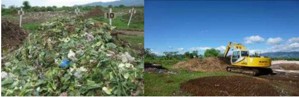
Piles of collected and transported green waste at the Vunato Waste Landfill, Lautoka, Fiji
