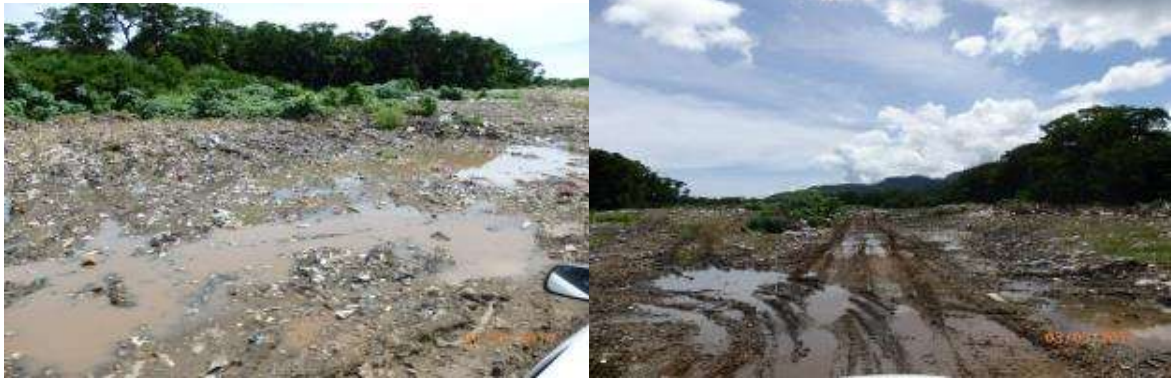
Usual waterlogged conditions of Namara Disposal Site, Labasa, Fiji
