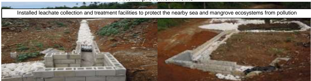
PVC Leachate Collection Pipes & Leachate Collection Pond at Kalaka Waste Landfill
