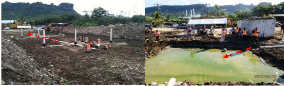
Improvement at the Pohnpei, FSM Disposal Site using PVC pipes and empty drums
