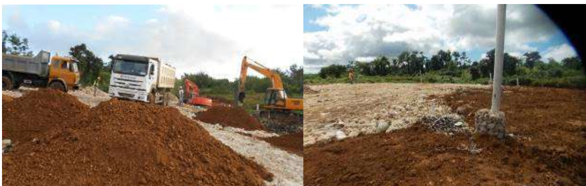
Supplying topsoil loads at the working face (left) & Clean look after soil cover (right)
