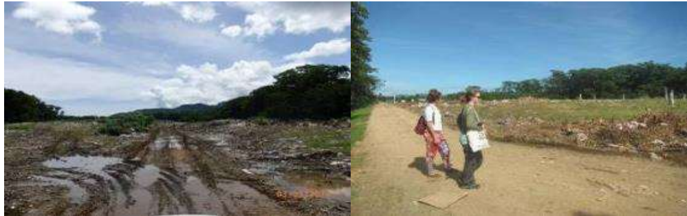
At the Labasa Dumpsite before (left) & road conditions after improvement works (right)
