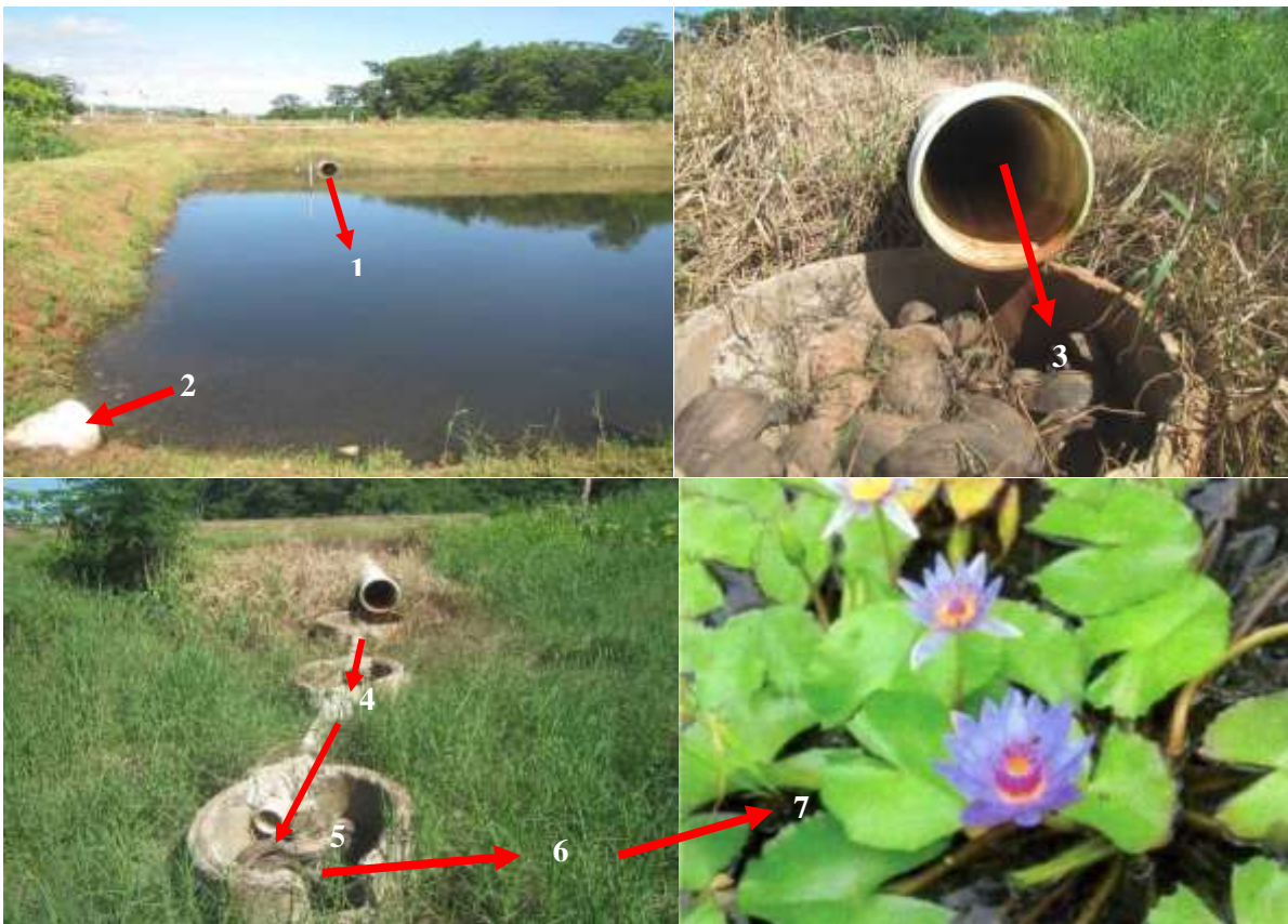
The Namara Waste Landfill Simple Treatment Facilities without any use of electricity
